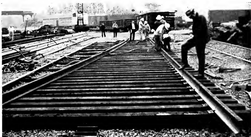
Jig for prefabricating turnouts at NYC's Alfred E. Perlman freight yard. More than 300 turnouts will be fabricated in this manner.
